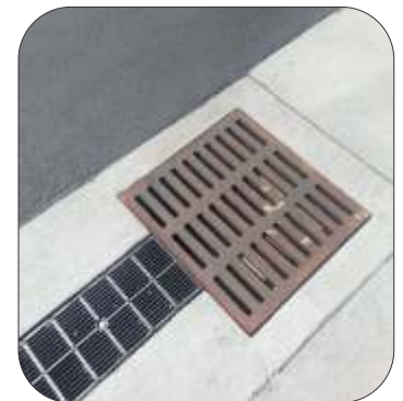
2' wide x 2' long x 4' deep basin at service station
